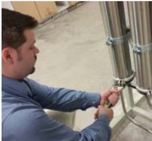
Reverse Osmosis Systems
